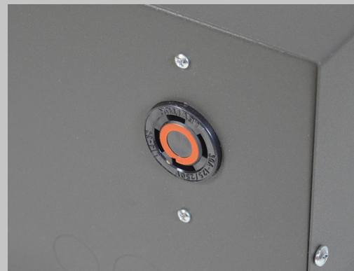
Twist-Lock Outlets and Plugs
