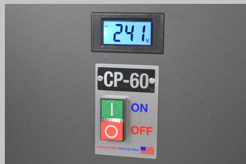
Digital Voltage Meter
